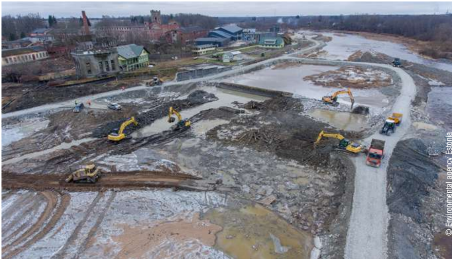
Removal of the Sindi dam, 151 metres wide and 4.5 metres high, on the Parnu River, a salmon migratory route, in Estonia in December 2018.
